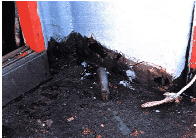
Photograph 1 Corroded accommodation house side structure
