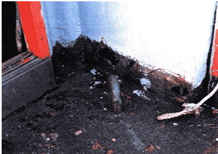
Photograph 1 Corroded accommodation house structure
