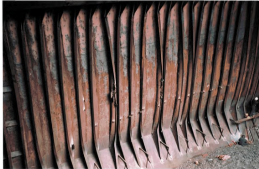
Photograph 1 Collapsed side shell frames (See Example 4)
