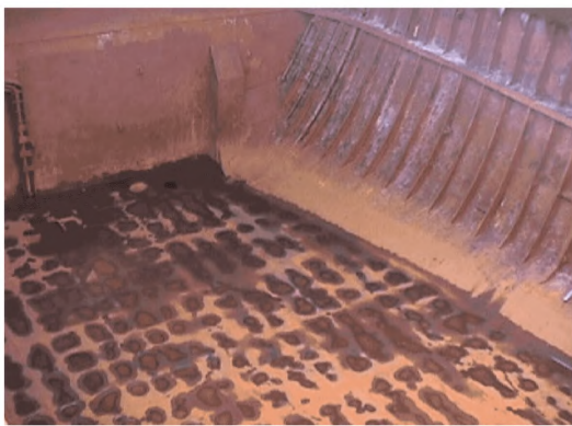
Photograph 2 Damaged inner bottom plating
