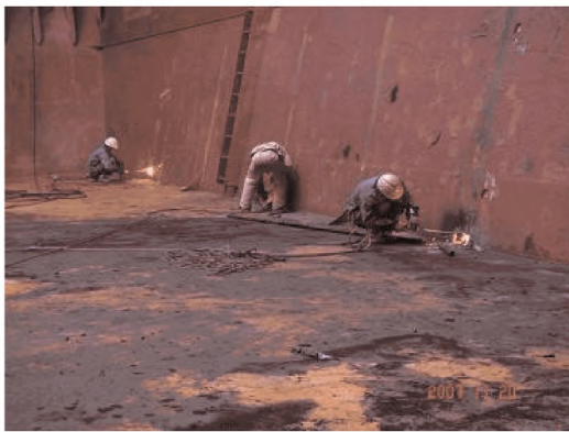
Photograph 1 Heavy corrosion affecting inner bottom plating
