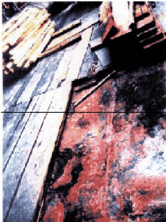
Photograph 1 Fractured inner bottom plating due to heavy corrosion on both sides
