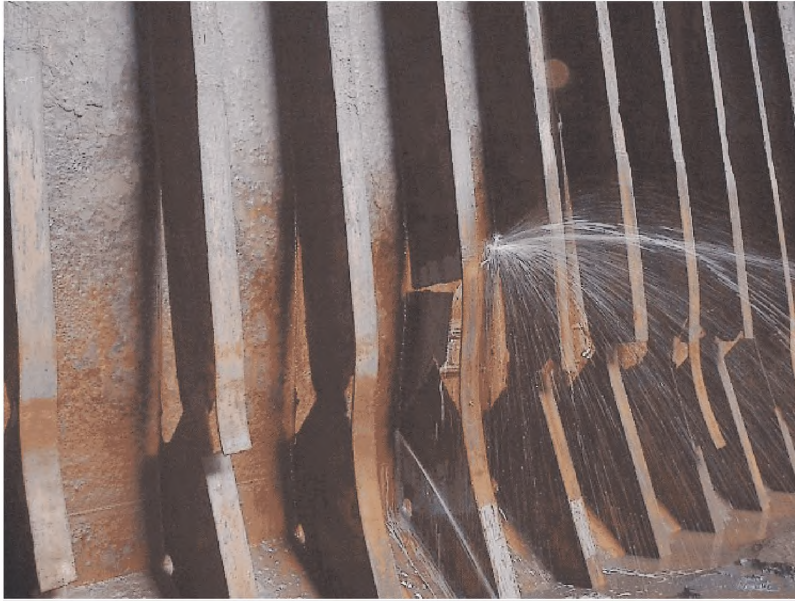
Photograph 1 Leakage from side shell plating due to heavy corrosion
