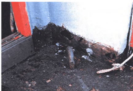
Photograph 1 Corroded accommodation house side structure
