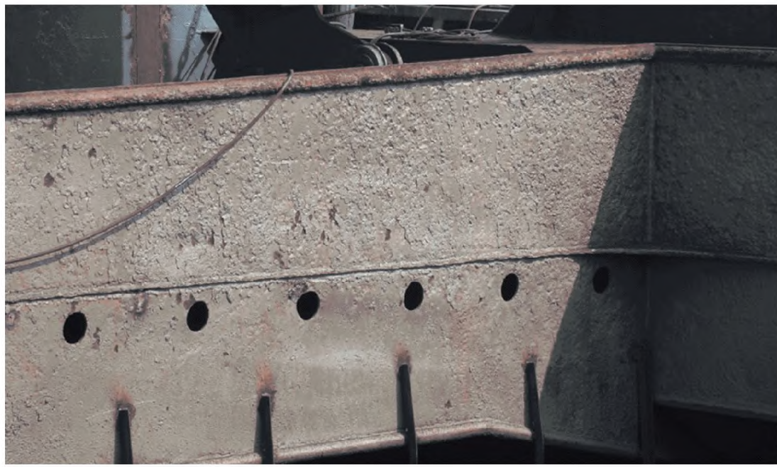
Photograph 1 Heavy corrosion of hatch coaming
