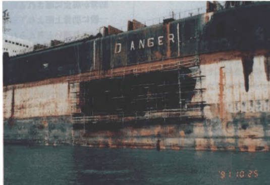
Photograph 2 Missing side shell structure (See Examples 4 and 5)
